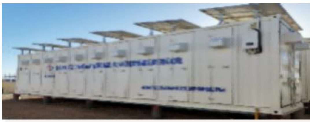
Guazhou, Gansu 12MWh Photovoltaic Energy Storage Project
