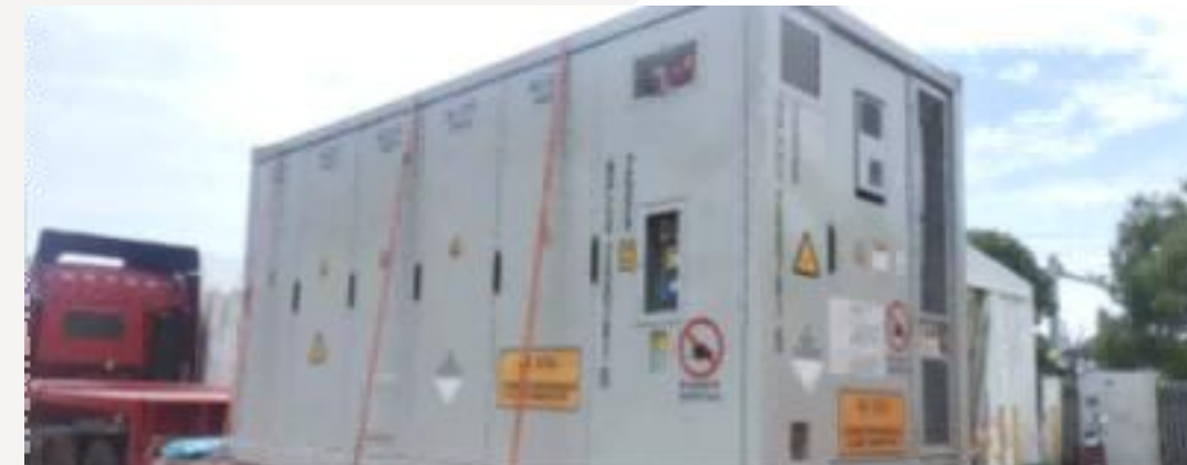
Bulgaria 7.45MWh photovoltaic distribution and storage
