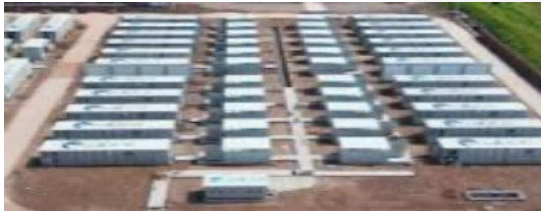
Chongqing Three Gorges Yongchuan 200MWh/400MWh
