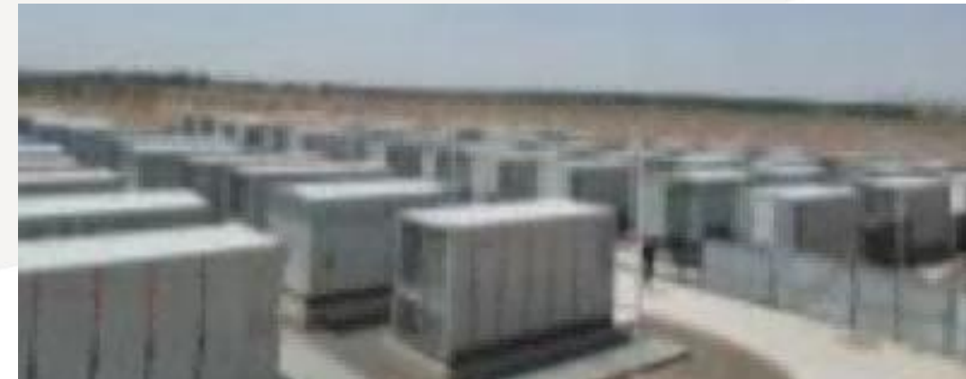
Belgium project 126MWh energy storage project
