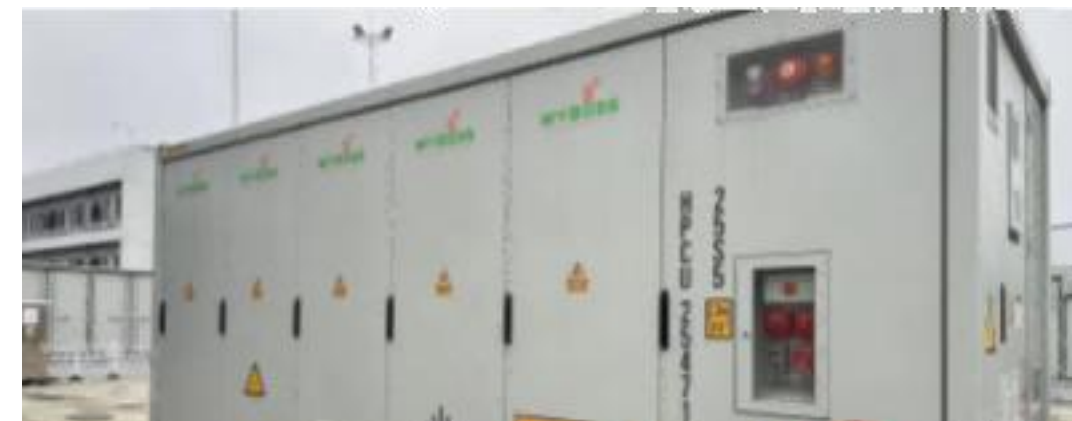
The 'MY BESS' project Malaysia sample 3.7 MWh
