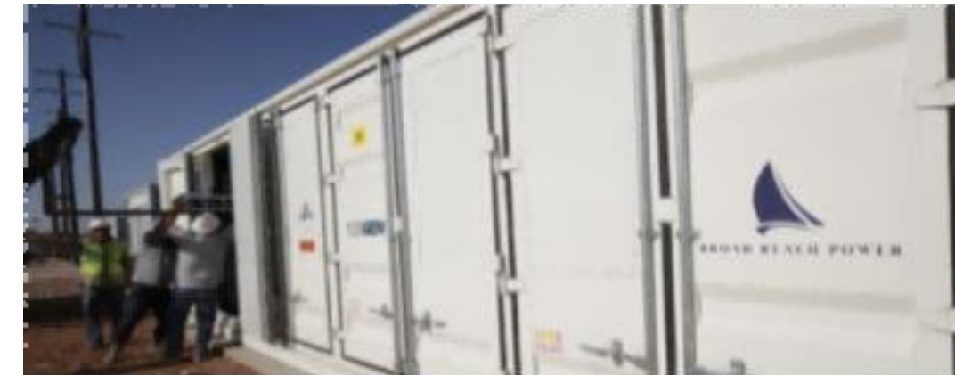
Cascade Energy Storage Project 117.5MWh California, USA
