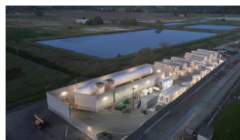
California, USA Calistoga Resiliency Center, 293MWh
