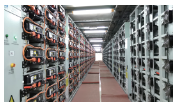
Morowali Industrial Park (IMIP), Indonesia 150 MWh
